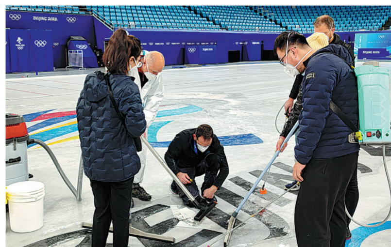
The Capital Indoor Stadium has installed an eco-friendly ice-making system that uses carbon dioxide as a refrigerant. XINHUA
